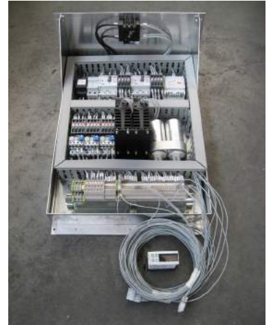
Rack 19" Standard electrical panel.
