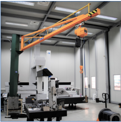
Roof gate opening for use of the external overhead crane and internal crane, for maximum flexibility
